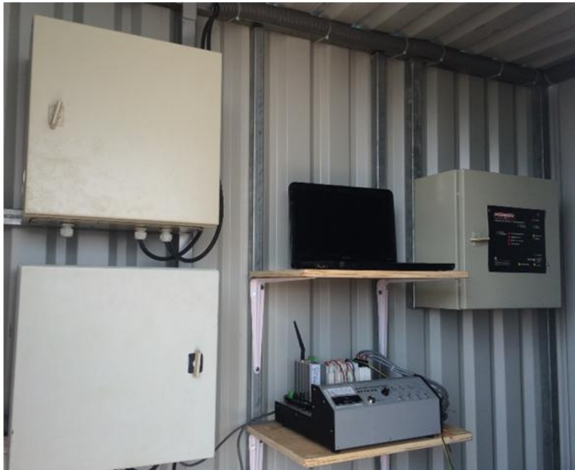
Figura 4.1 Cabina de control instalada
